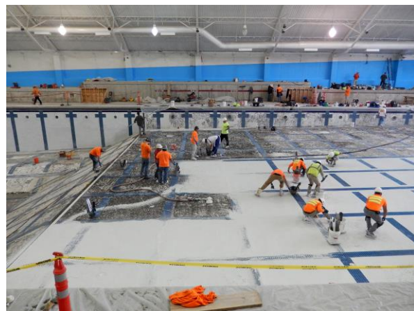
One of the top priorities of the improvement project was to resurface the plaster pool tank. The Olympic-size pool measures 50 meters long and 25 yards wide.
